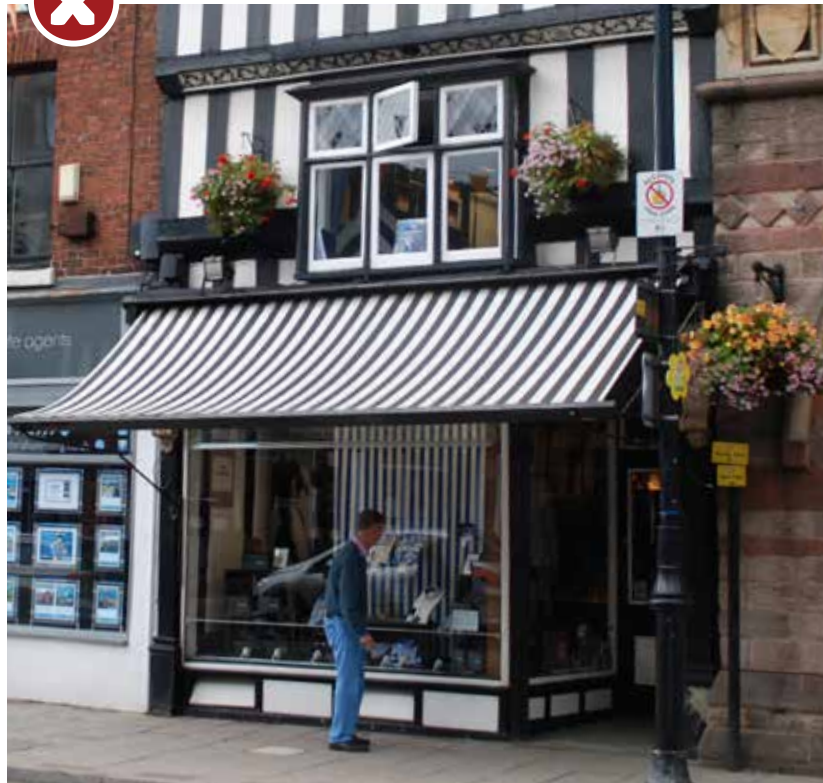
Figure 65: Flat shopfront insert and undivided glazing detracts from the existing traditional frame and the character and appearance of the host building.
