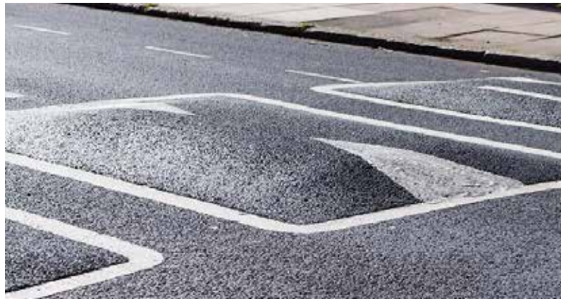
Figure 32: Traffic calming bumps
