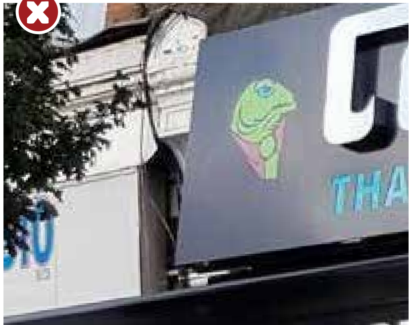
Figure 71: Bad example of a pilaster treatment. The original detailing is covered by bulky fascias.
