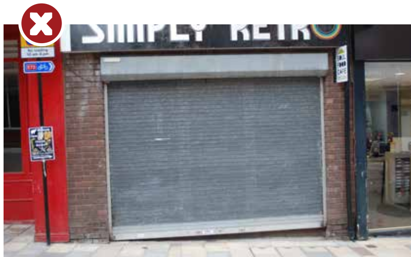
Figure 80: Solid shutters are not acceptable
